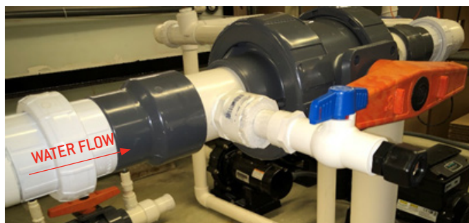
Inlet water pitot tube - notch facing downstream
